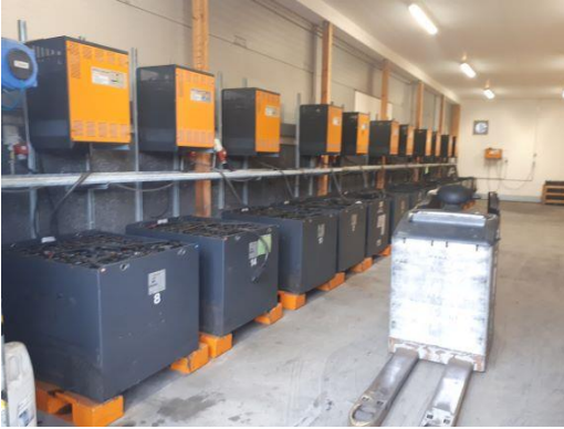
Ladestation for el-gaffeltrucks.
