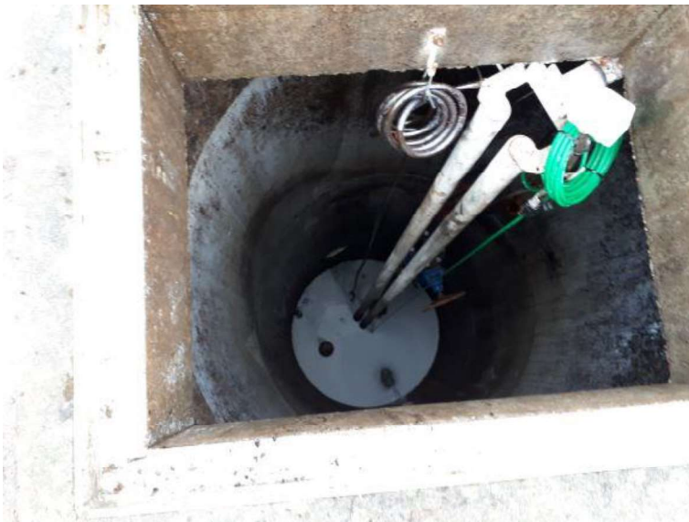
Pumpebrønd for spildevand
