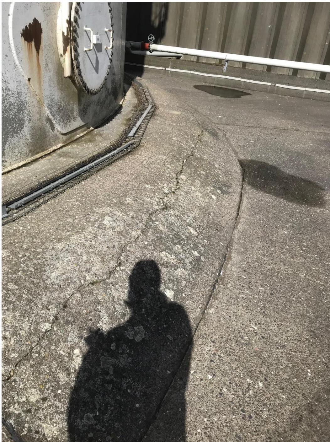
Tank 57, revne i tankpude
