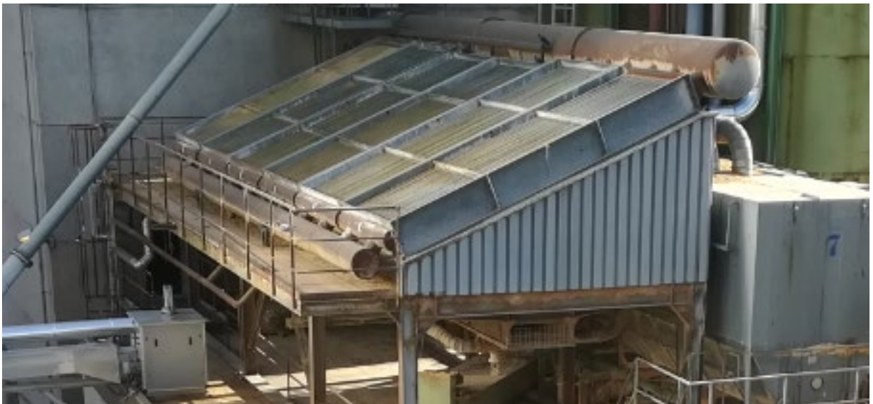
Existing Balance Cooler
