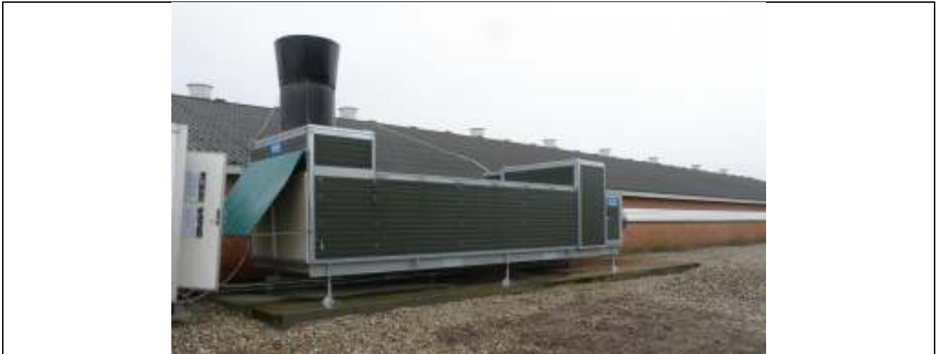
Figure 1. Picture of the Agro Clima Unit situated outside the test broiler section. Ventilation air to and from the broiler house are drawn through the Agro Clima Unit by a counter current principle to utilise the heat content of ventilation air to heat up inflowing air.
