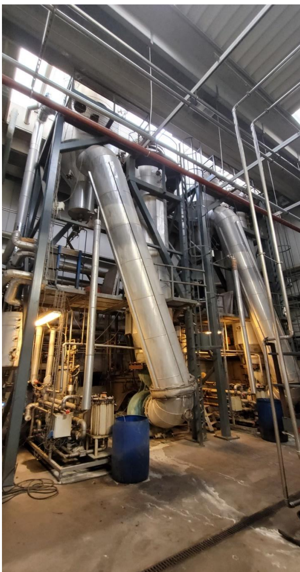
De to inddamper kolonner.
