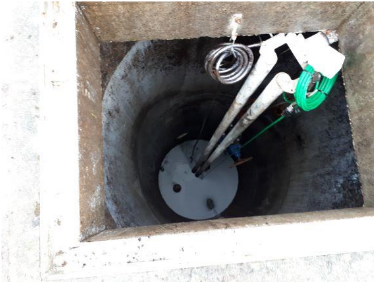
Pumpebrønd for spildevand
