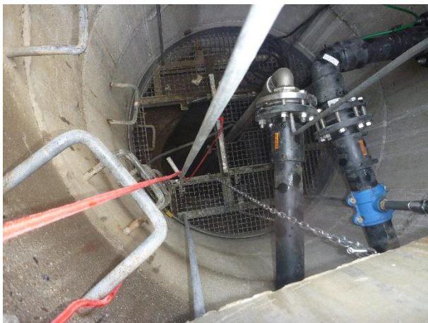
Figur 4: Pumpebrønden i Deponi 2.
